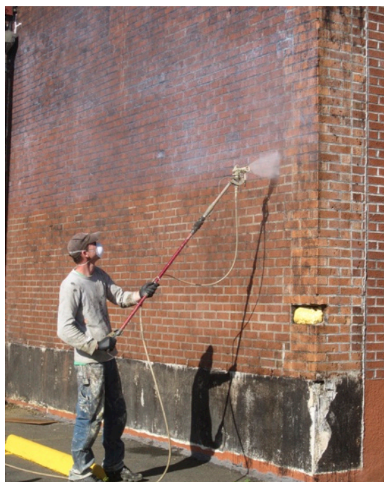
In late fall, Lincoln City Urban Renewal Agency began work on the repair and restoration of the south wall. Above, a local painting contractor applies sealant to the newly-exposed brick.
